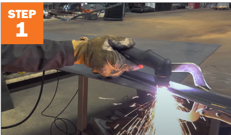
Plasma cut the sides. Tip: clamp down a metal straight edge as a guide
