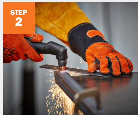
STEP 2 Cut tubing and angle iron to length. Then cut a 45-degree angle in top four edges of angle iron.
