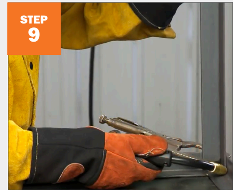
STEP 9 Tack legs into corner on the inside of the frame to hide corner welds.
