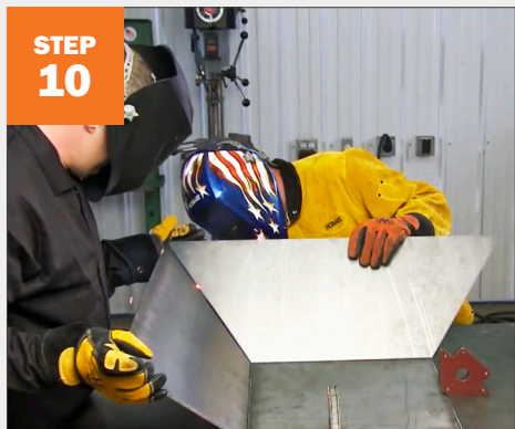
STEP 10 Begin building the fire box by placing the bottom square on the table and tack weld each side of the box. Tip: When placing the sides of the fire pit together you are going to want some assistance holding up the sides.
